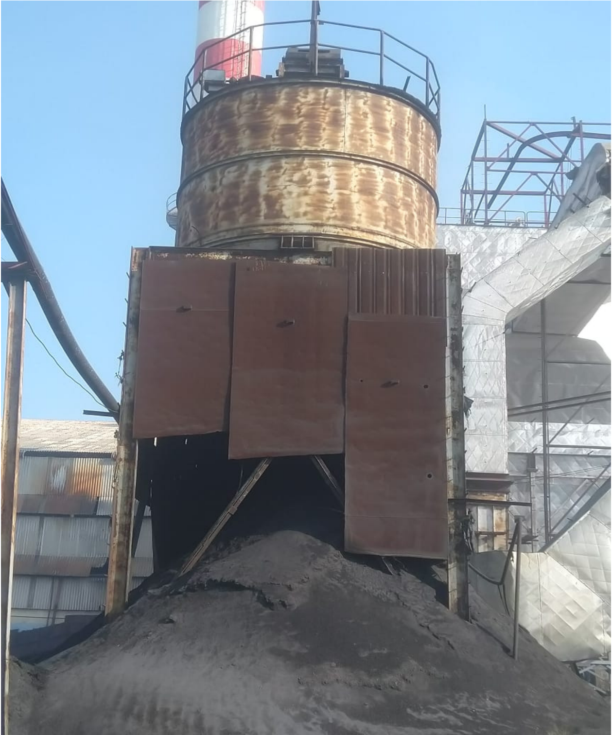
Photograph showing Silo for bottom ash collection
